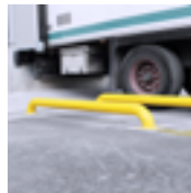
DOCK WHEEL GUIDES
