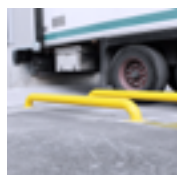
DOCK WHEEL GUIDES
